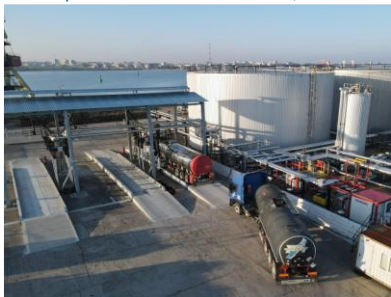
Terminal de Bitum MANGALIA Capacitate stocare bitum: 25,000 m 3
